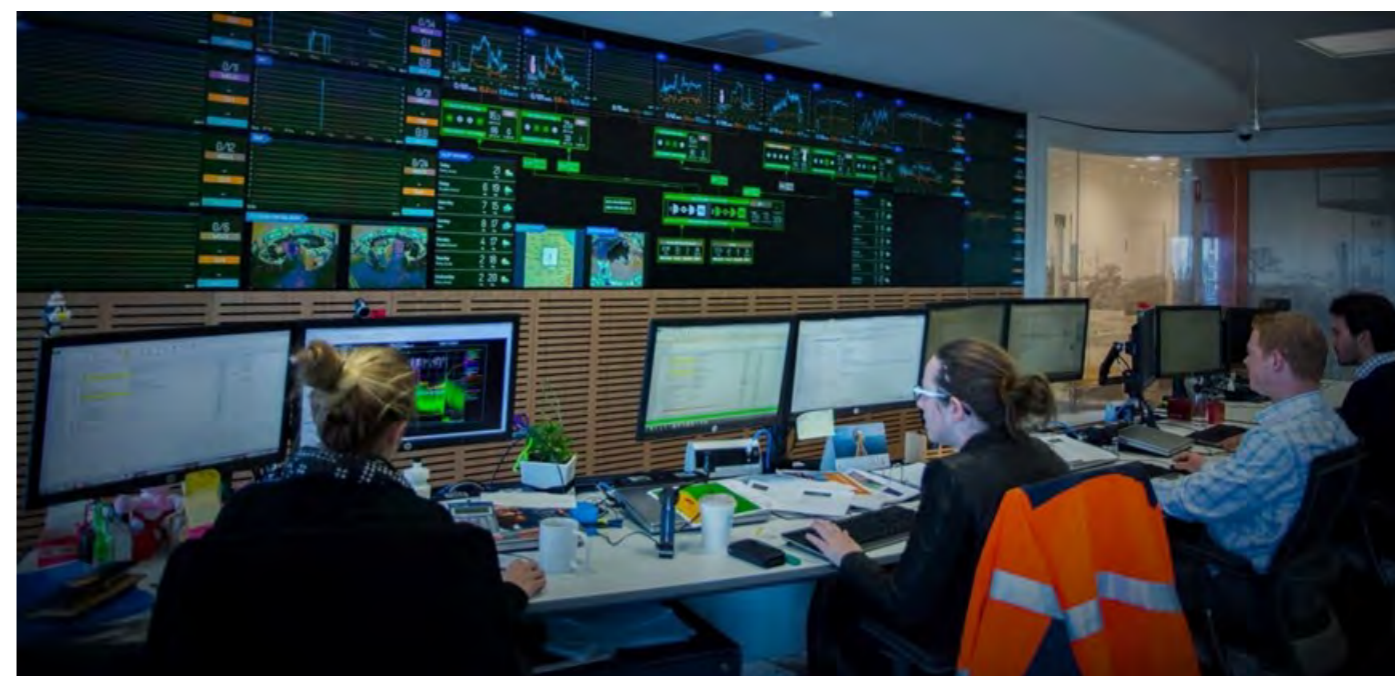
Figure 2. Large Surveillance room for monitoring of tight gas field, pipeline system and LNG plant
