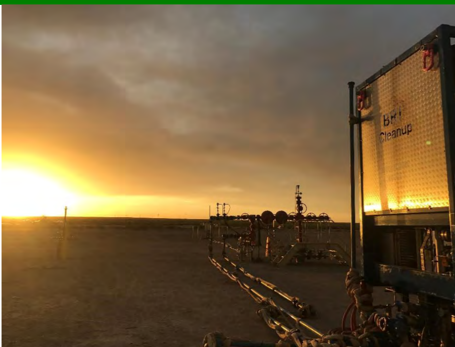
Figure 4. BRI Cleanup Dynamic Desander unit in unconventional fracking operation in USA.
